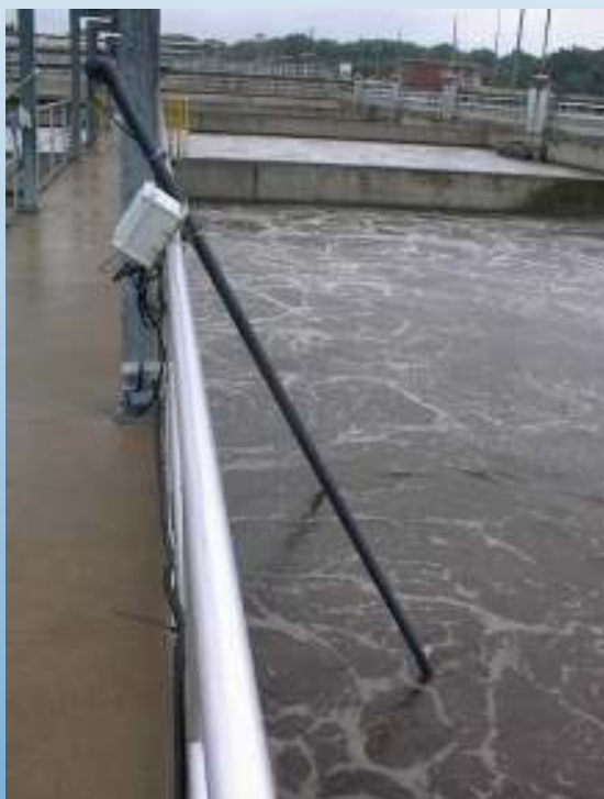
Diffused air Activated Sludge Plant monitoring and control
